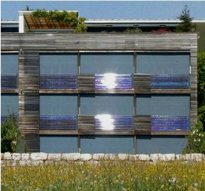
Façade integrated evacuated solar collectors (Sunny Woods, arch. Beat Kämpfen)
